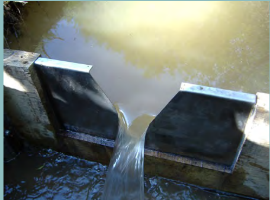
Figure 41. Notch weir flood control. Source: eDesign Dynamics.
